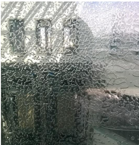
Figure 2. Delamination of fire resistant glass filled with sodium silicate gel
