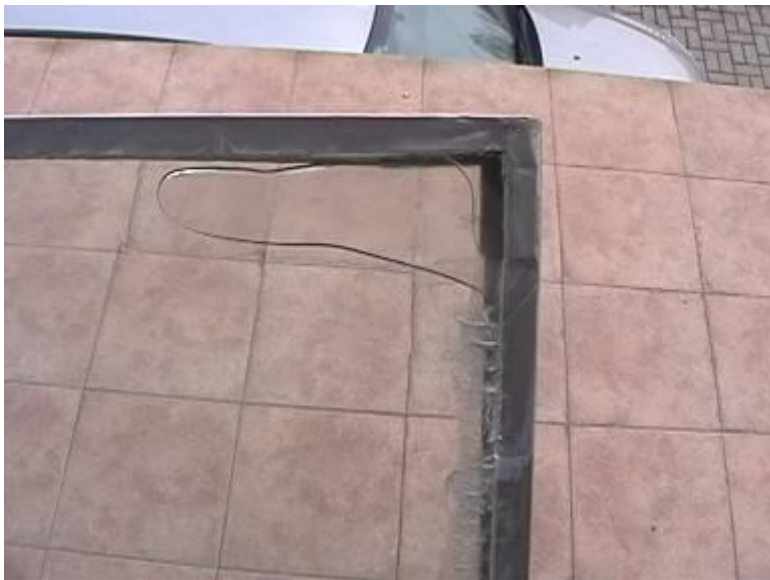
Fig 1. Air cavities in Pyrobel glass, resulted in breakage of peripheral insulation and penetration of water.
